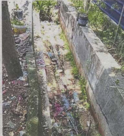
Drains in bad condition along Jalan Lama Port Klang. The water cannot flow due to clogged drains.
