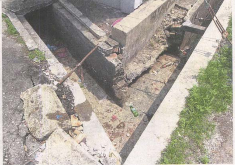
A broken drain in the Taman Chi Liung commercial area.
