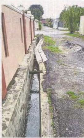
Broken drains and sinking roads along Lorong Bagor in Taman Petaling Indah Klang.
